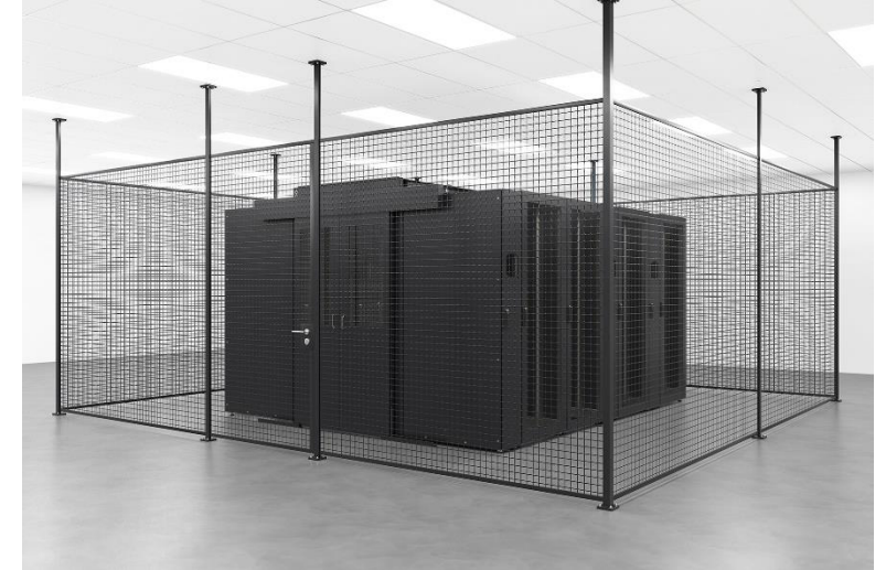
Rack Space 47- Caged
